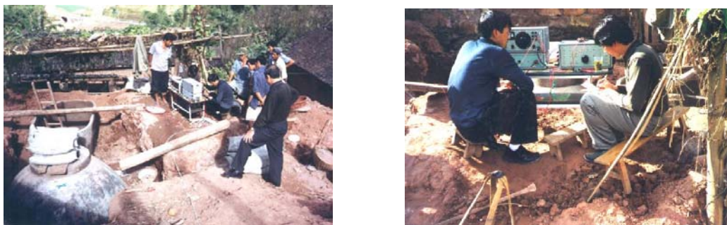
Fig. 4 Testing field of structural deformation of biogas digester constructed of bamboo-woven concrete
