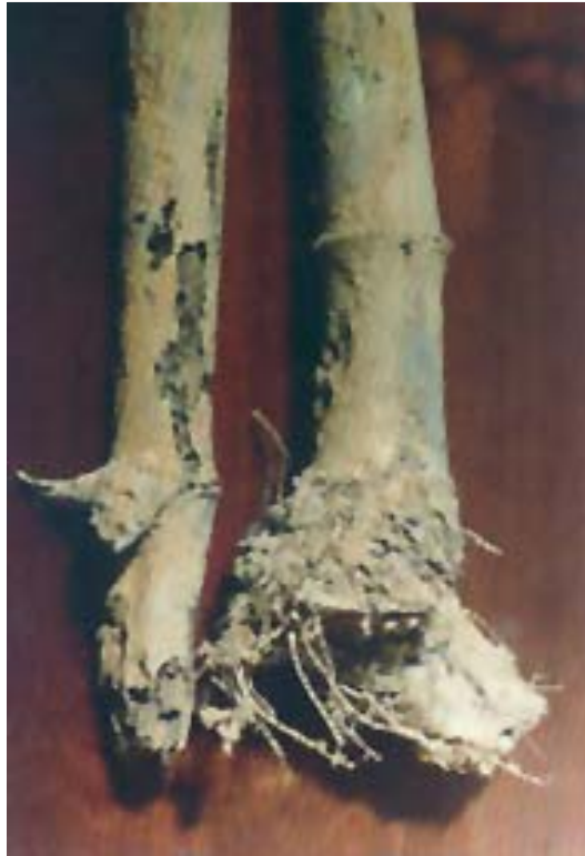
Fig. 53: Damage caused by termites
